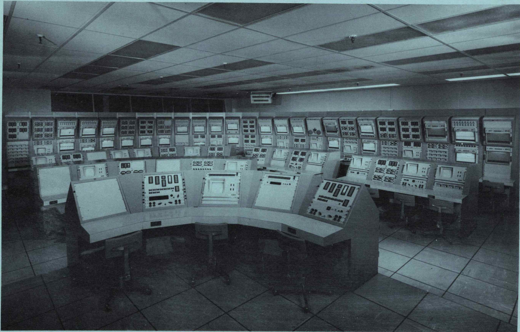
Figure 1. ACE-S/C Control Room
