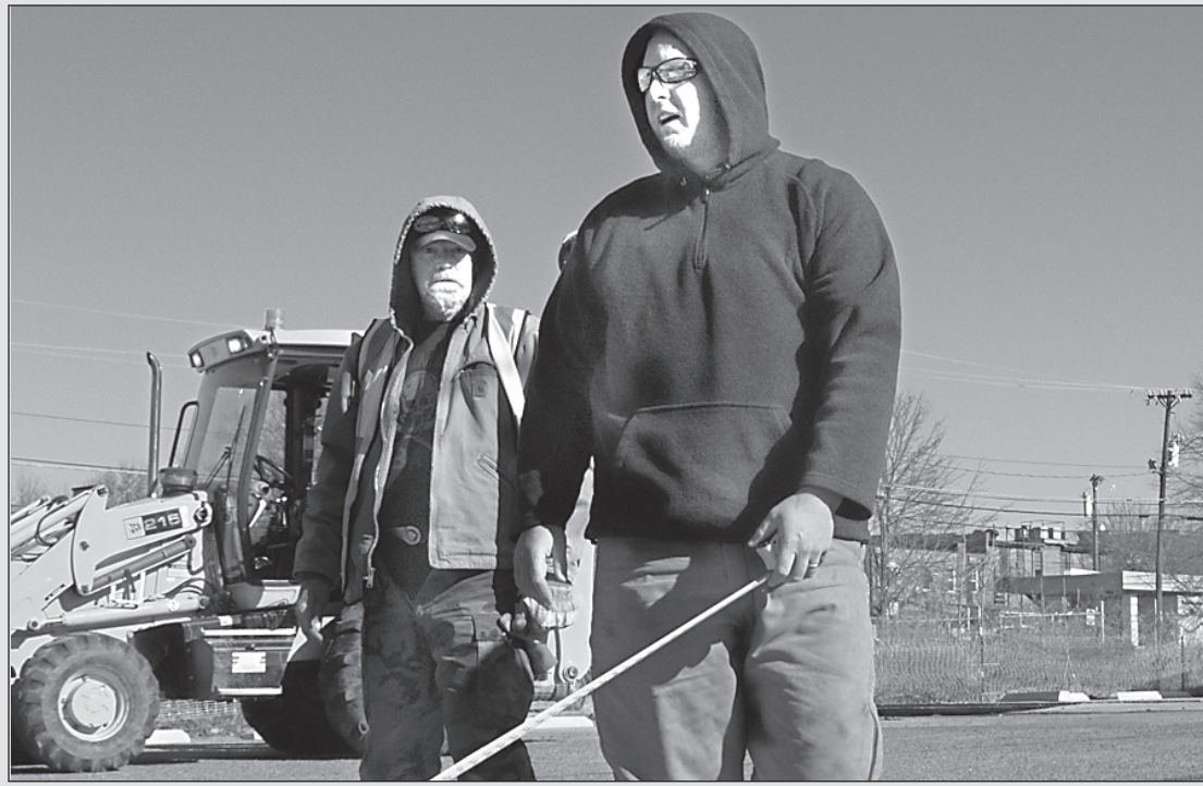
Chilly weather hasn't stopped work on downtown Carrboro's newest public parking lot. Manuel Turner and Chad Dusenberry work on marking off some of the roughly 90 spaces soon to be available at the corner of Roberson and Greensboro streets.
