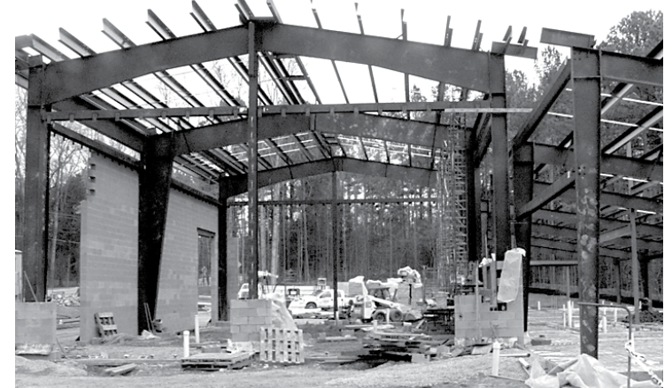
PHOTO BY KIRK ROSS Carrboro's new fire station under construction on Homestead Road.
