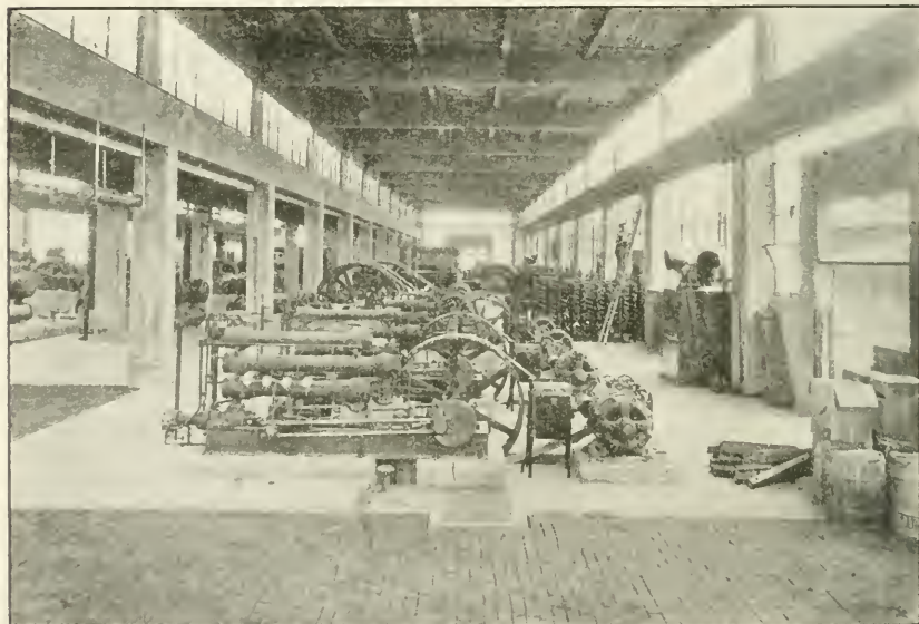
Interior view, compressor building, United States Helium-Production Plant, Fort Worth, Texas.
