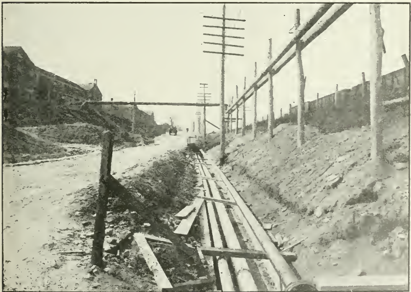
Elevated and underground distributing systems, Submarine Base, New London, Conn.
