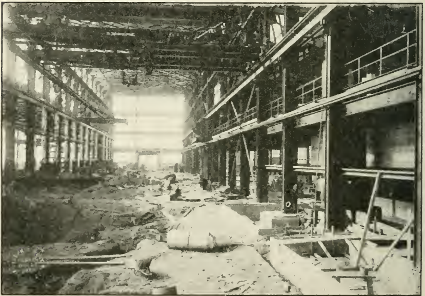
Foundry, Navy Yard, Philadelphia, Pa. Interior view.
