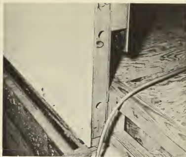
Figure 19. Panel at Floor Level
