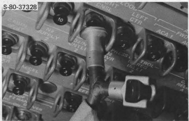
PUSHING CIRCUIT BREAKER
