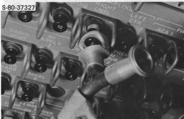
PULLING CIRCUIT BREAKER
