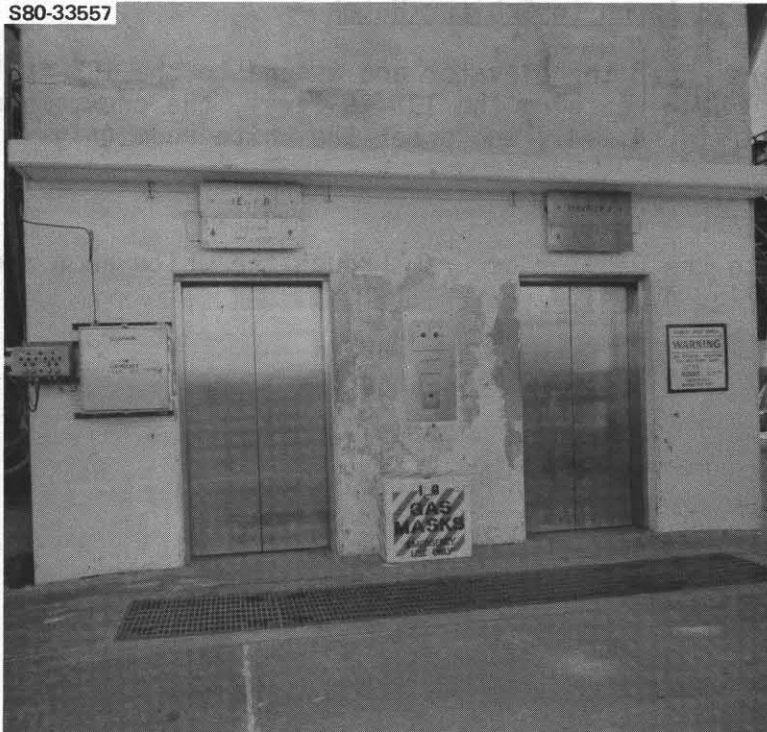
ELEVATORS - GROUND LEVEL
