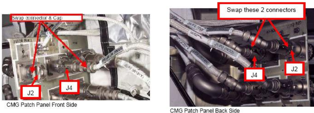
Figure 3-38. Z1 Patch Panel
