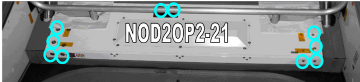
Figure 7. Radial Bay looking Overhead-port. Locations of bolts apply to all other appropriate areas in Radial Bay.
