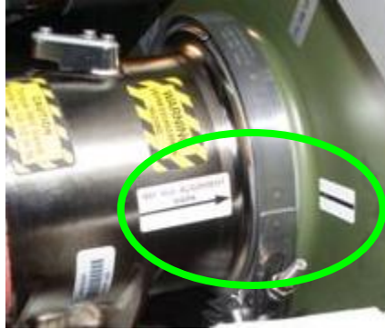
Figure 14.- Typical IMV Valve Reference Marks in Node 2.
