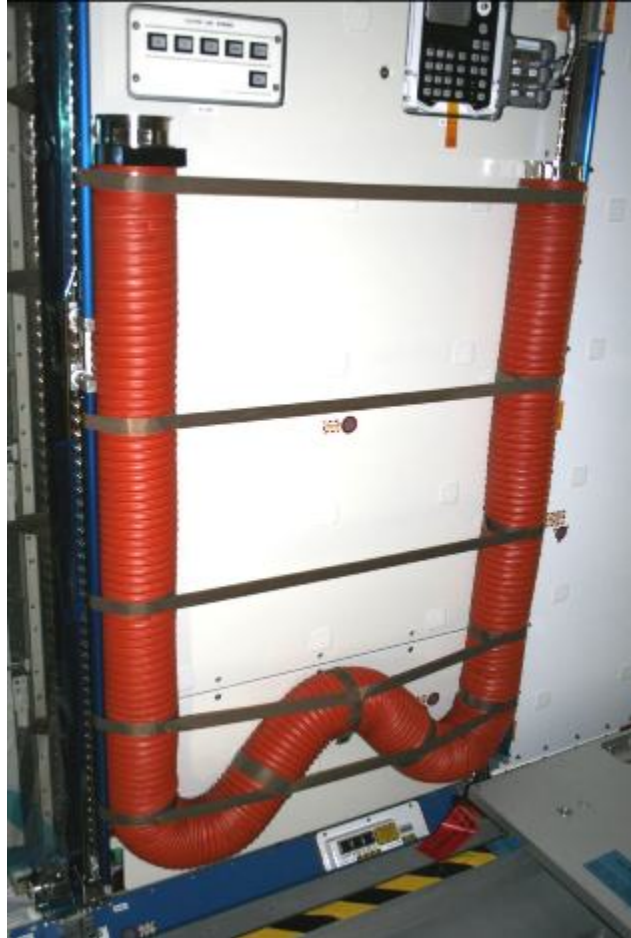
Figure 8.- Flexible Ventilation Duct (13 ft) stowed in Node 2 (launch configuration).
