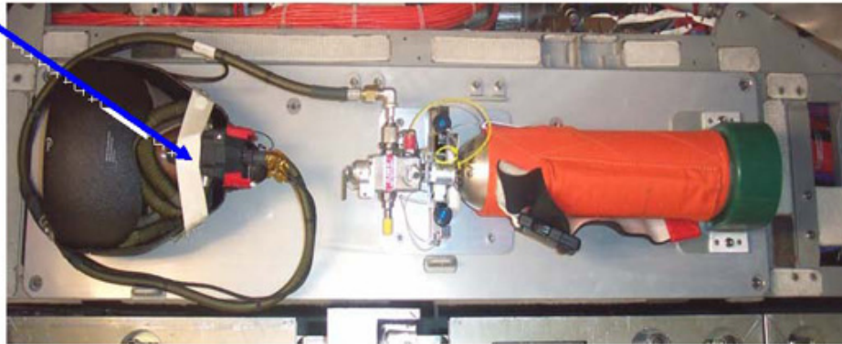
Figure 3-2 PBA1(2) at Installation Location (Protection Covers not installed)
