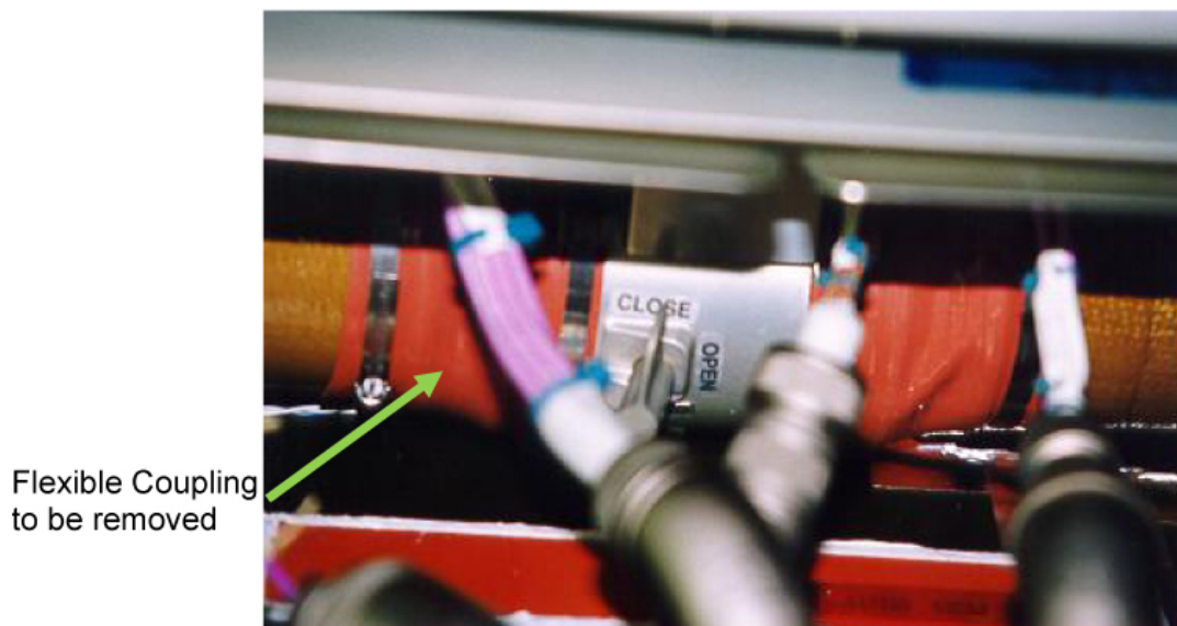
Figure 17. Node 1 Duct Valve 4 (Located at NOD1OP2).
