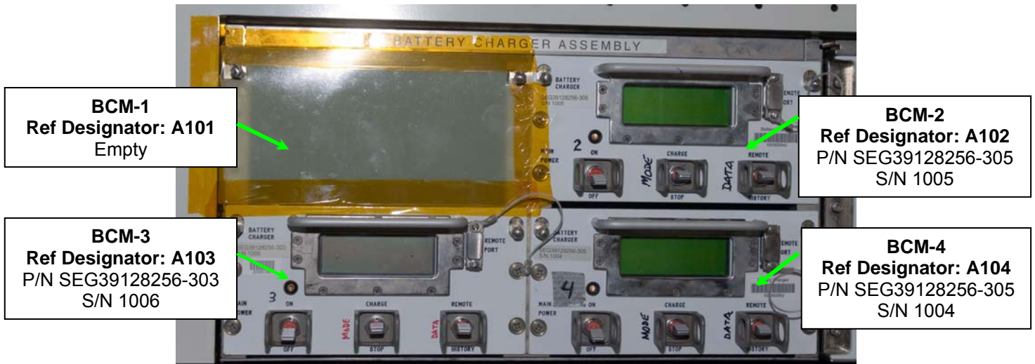
Figure 1.- Battery Charger Module Reference Designations and Current Configuration.
