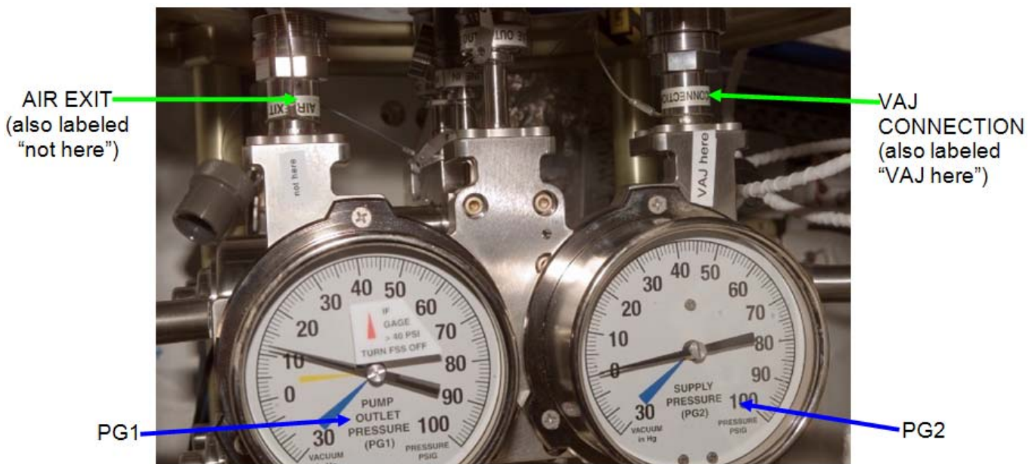
Figure 2.- AIR EXIT and VAJ CONNECTION on FCPA.
