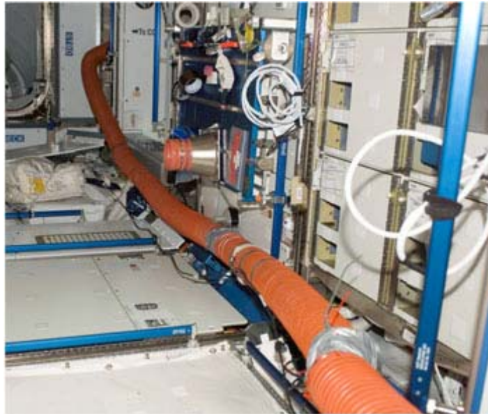
Figure 3.- Node 2 Temporary Duct Routing.
