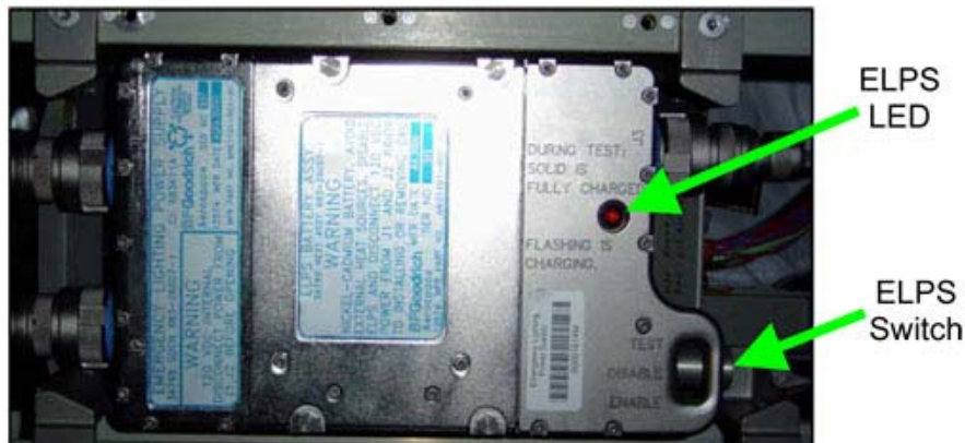
Figure 2.- ELPS Switch Location.
