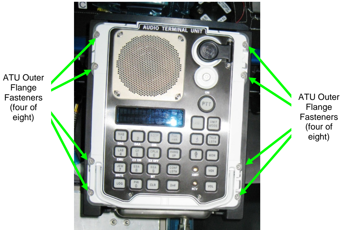
Figure 6. - ATU Outer Flange Fasteners.
