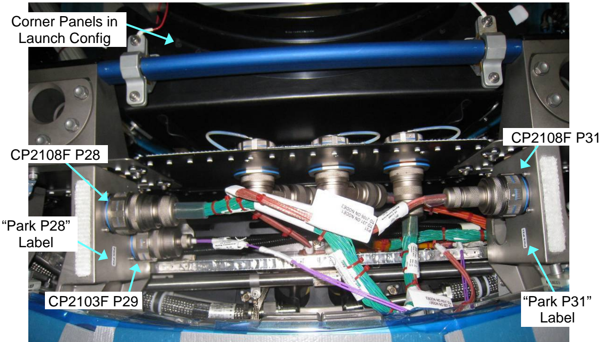
Figure 18.- Cupola Fwd Quadrant Dummy Connections.
