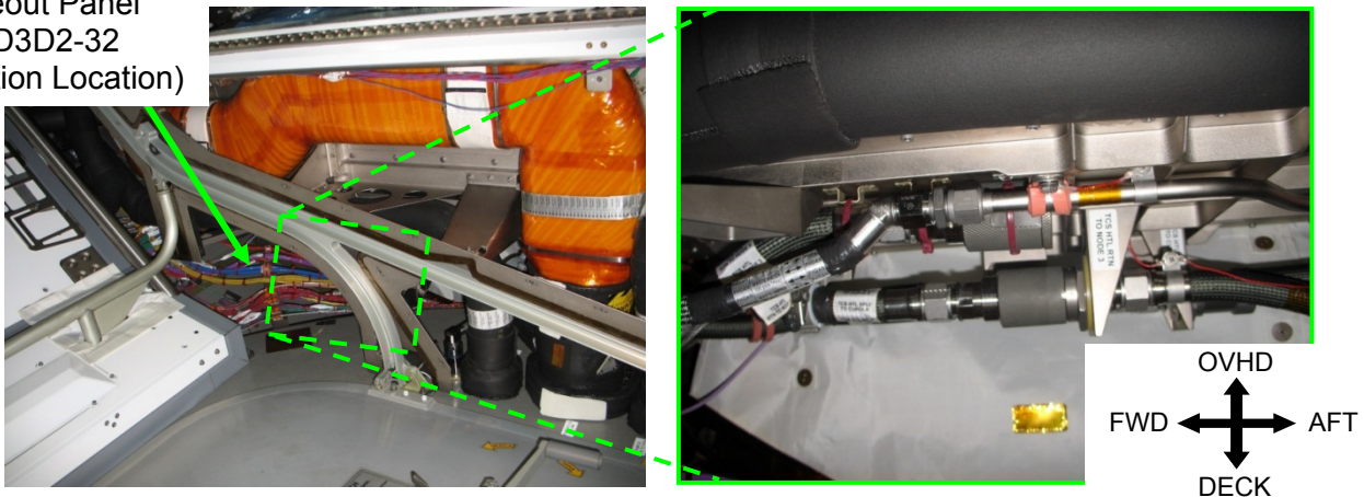
Figure 7.- Cupola HTL QDs in Node 3 Deck Midbay (looking Starboard).
