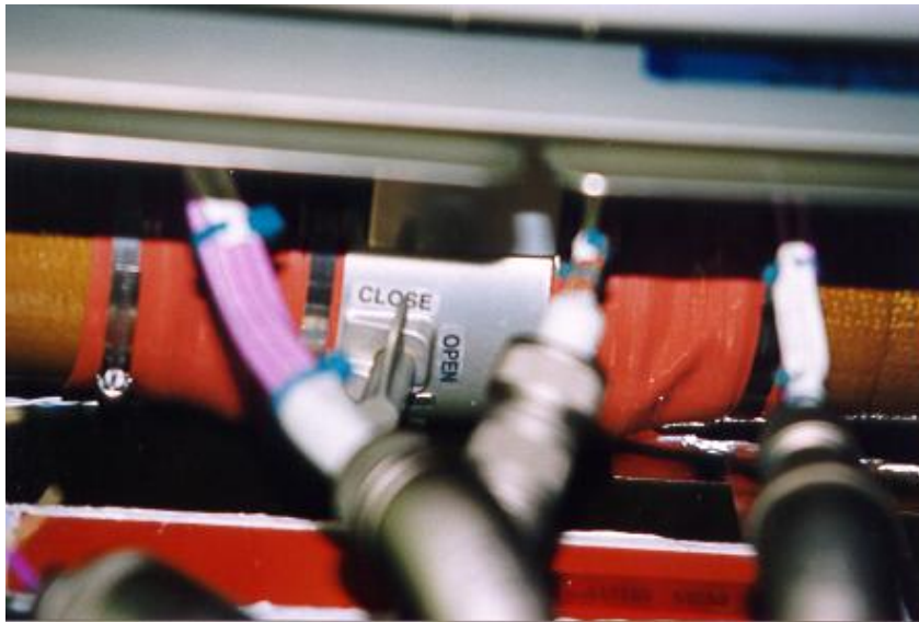
Figure 17.- Node 1 Duct Valve 4 (Located at NOD1OP2, View Looking Zenith).
