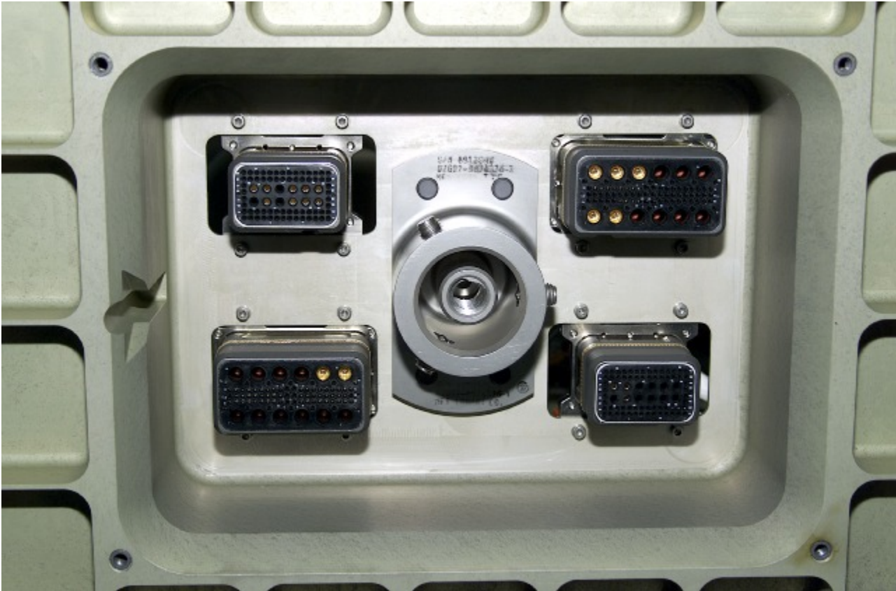
ECU Installation Area on P6 SAW
