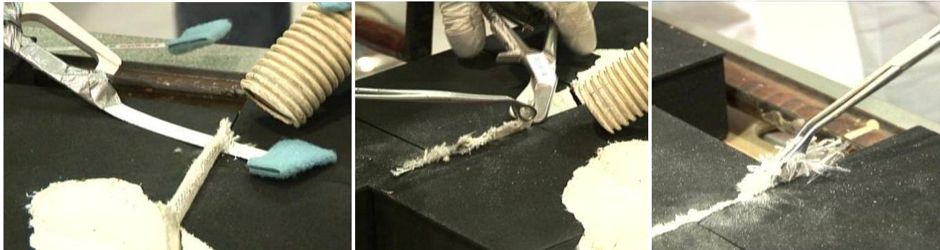
Figure 5 – Cutting pillow gap filler may require several steps before the area is completely cleaned up
