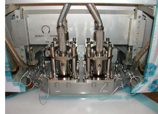
PVR FQDC – NOTE “B” and “A” Labeling incorrect
