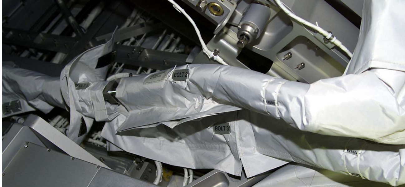
Figure 1.- Hose box P-clamps have labels with bolt numbers.
