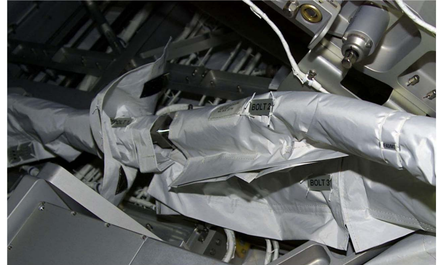
Hose box P-clamps have labels with bolt numbers
