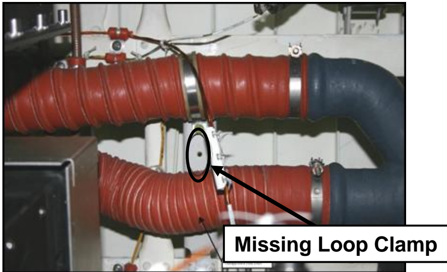
Avionics Bay 1 Ducting
