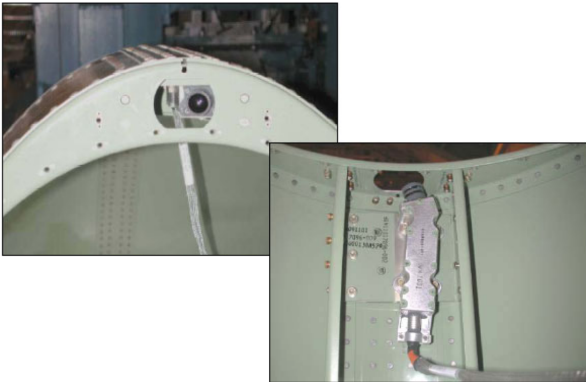
Figure 78-6. Camera Installed in Feedline Fairing
