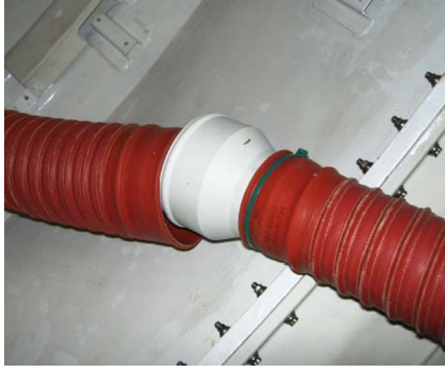
Figure 1-3.- Airlock/Tunnel Adapter I/F Duct reducer removal (view looking aft into Tunnel Adapter from Airlock)
