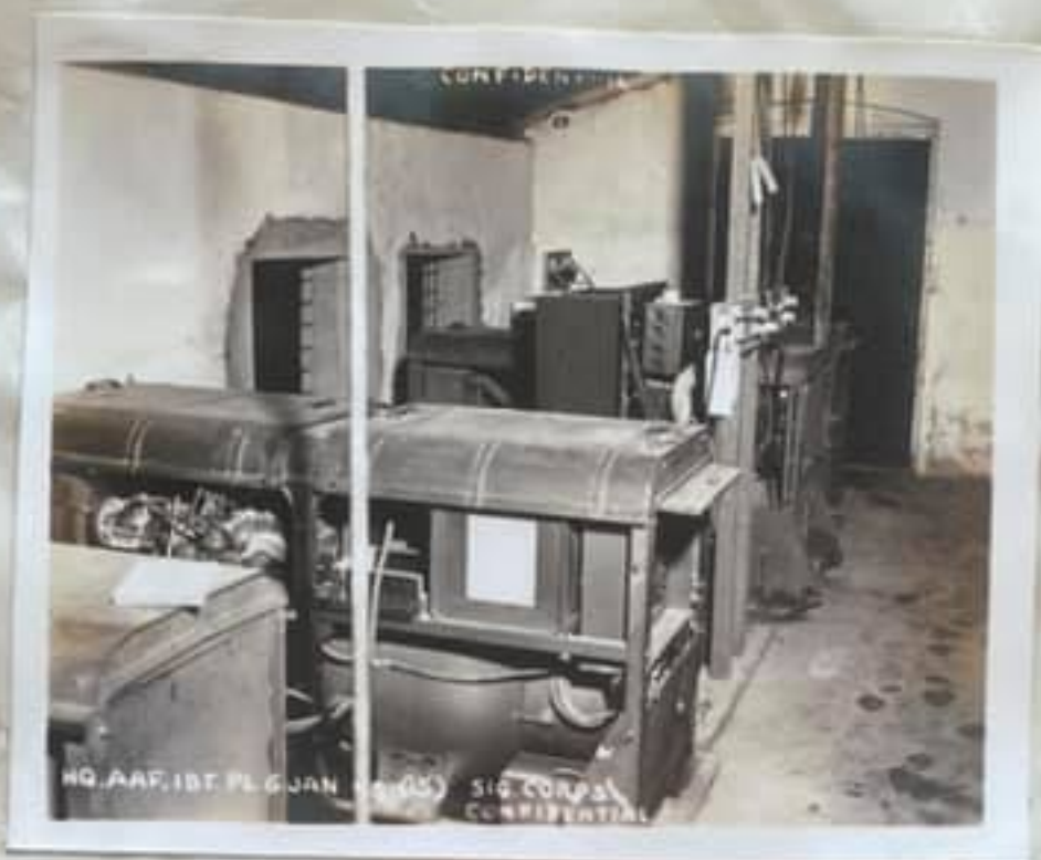
POWER ROOM -- The Power Room, situated directly opposite the East wall of the 424th Signal Center, houses the gas driven generators which provide emergency power for all signal equipment operated by communication personnel of the 424th Signal Company, Aviation.
