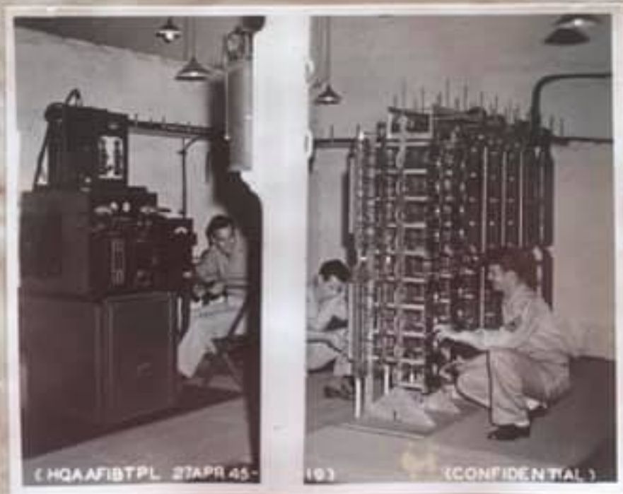
TELEPHONE MAINTENANCE ROOM -- W/Mgt Frank H. Wilcox, Wire Chief, and his assistants, S/Mgt Polnin, left, and T/A Sylvester, center, in the maintenance room of the Telephone Exchange. On the left is shown the power panel and test desk with the fire extinguisher up above ready for emergency use. On the right is the power frame (M-19), supplying full power for the switchboards behind the left wall.
