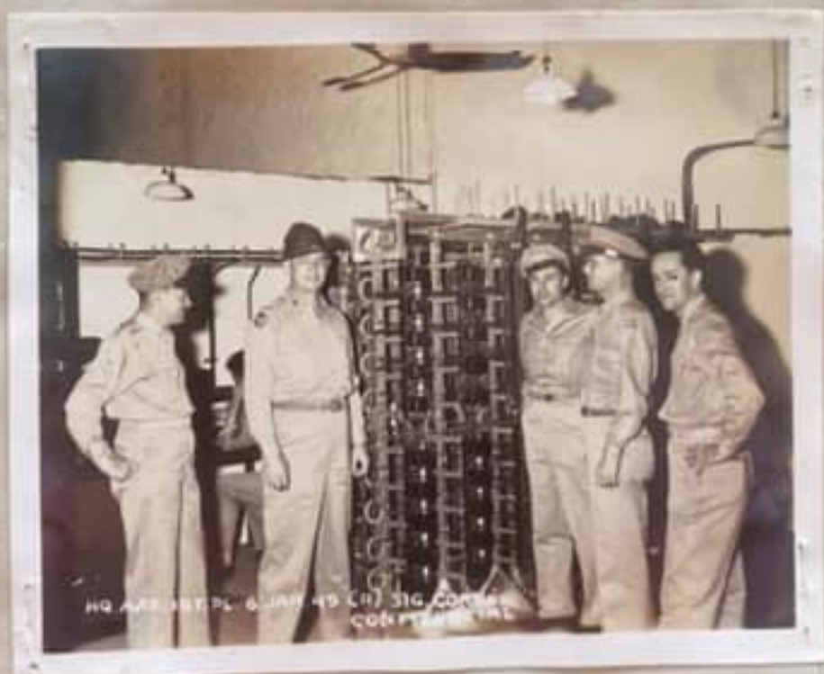
INSPECTED -- Inspecting the power frame situated in the Power Room directly behind the Telephone Switchboard, "Buffalo Exchange" area, from l. to r., First Lieutenant HENRY A. HEINTZEN, Captain OWEN F. HAYNES, Major ALFRED H. SCHMIDT, Base Executive Officer, Col CARL L. JENSEN, Commanding Officer, Hastings Air Base and First Lieutenant JOHN F. O'BRIEN.
