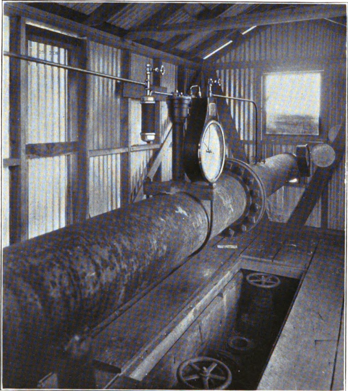
Fig. 11—ORIFICE METER ON LARGE GAS MAIN
