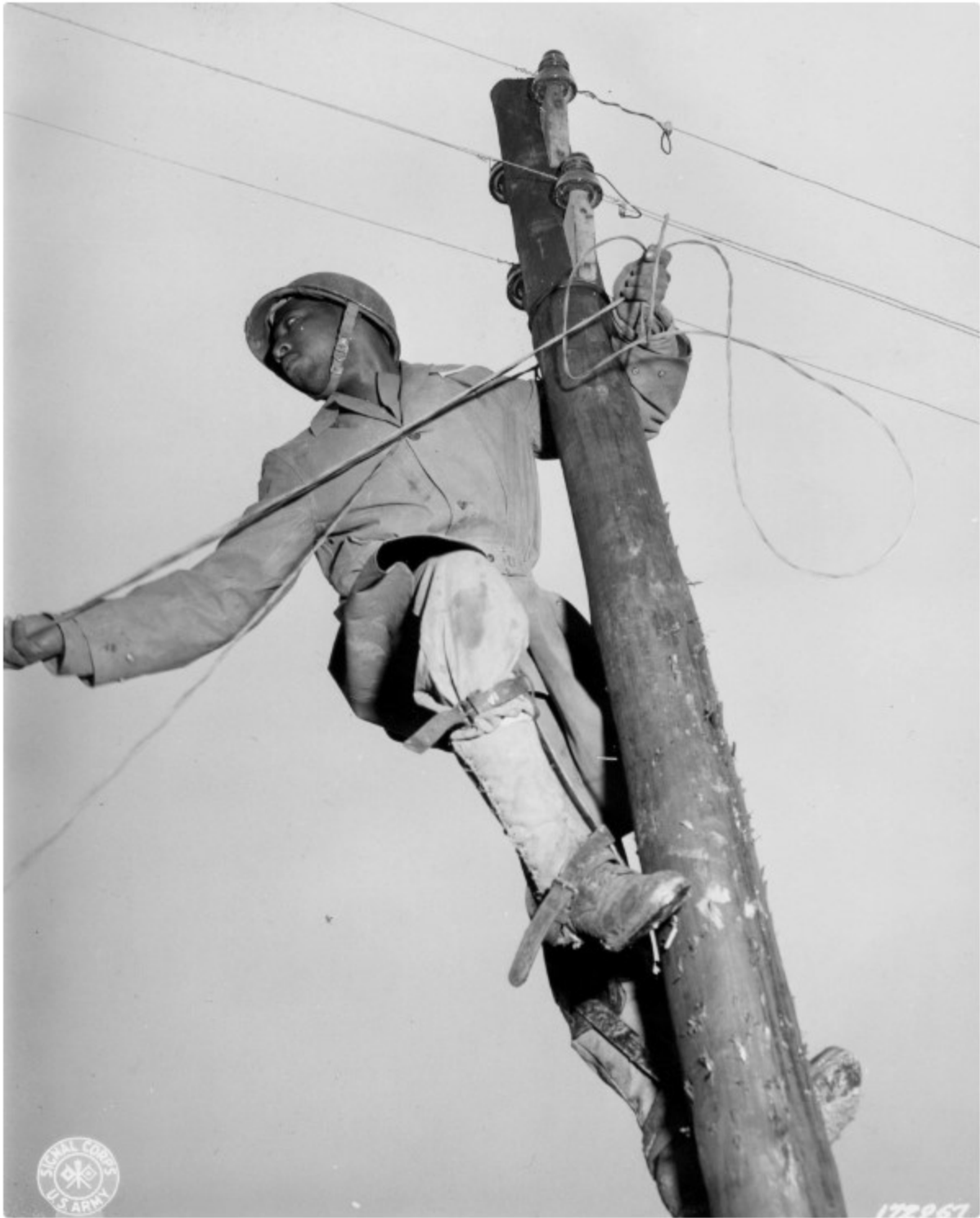
Pfc. Stanley Strickland of 93rd Signal Construction Co Marietta, Georgia strings wire for Red Army during Third Army Louisiana Maneuvers, Camp Polk, La. 4/18/43.
